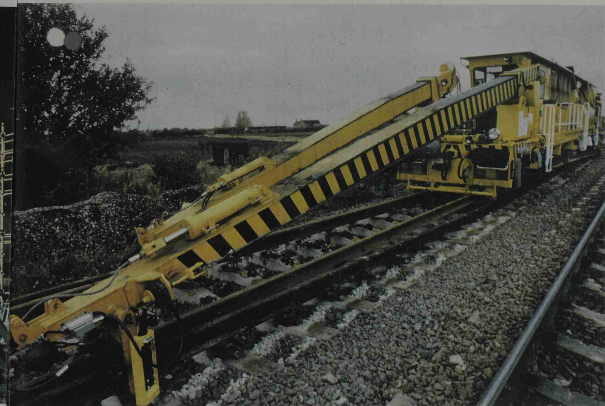
Rail Changing Machine in action, substituting long welded rails for jointed track.
