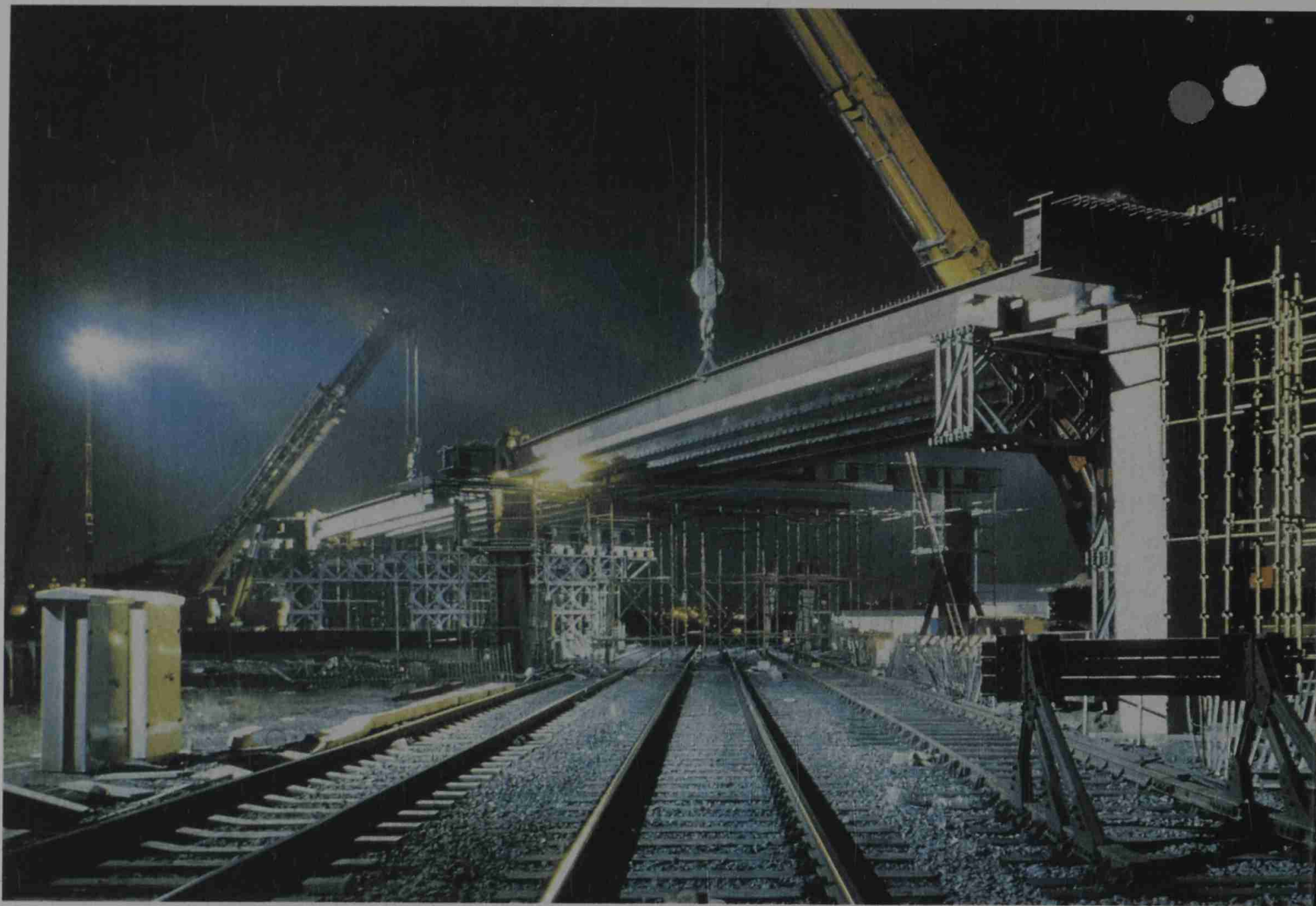
Major road improvements in the U.K. Carried out without interference to rail traffic.
