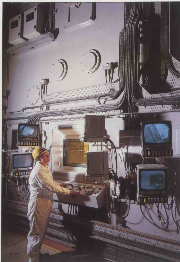
An operator outside one of the inlet cells.
