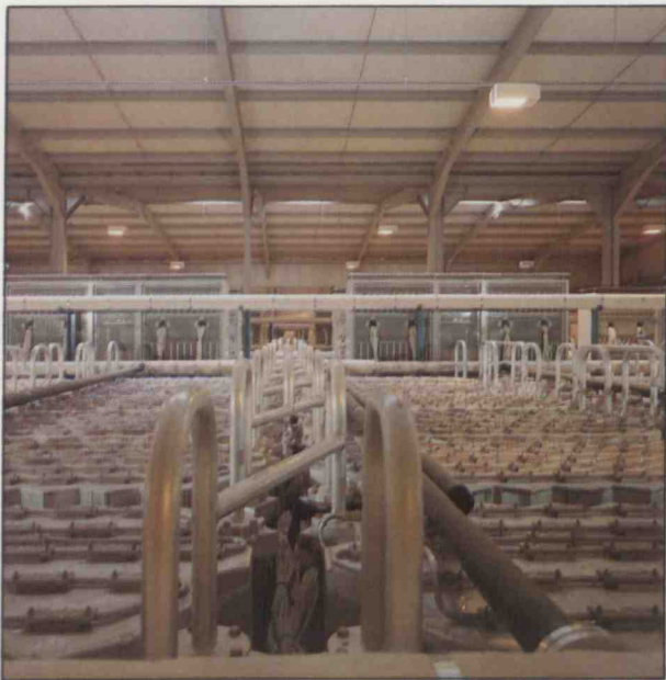
View across the top of a centrifuge cascade.
